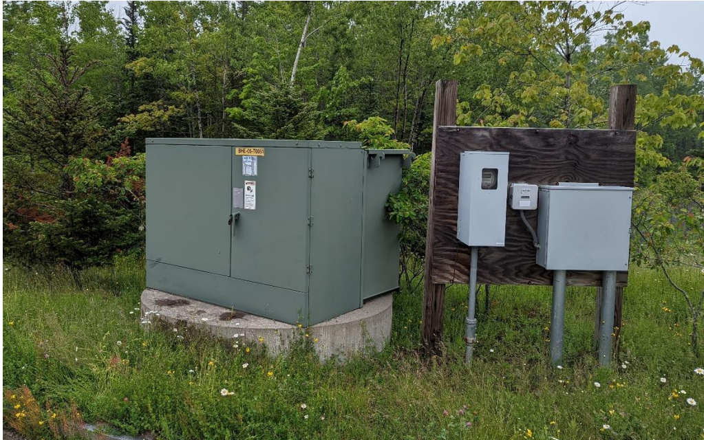
Figure 17 Existing Transformer at the Depot
